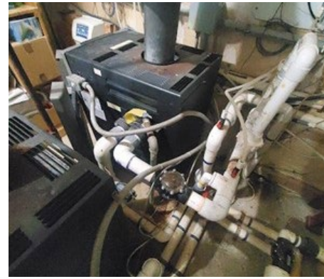
The rust stains around the vent stack are a strong indicator that the interior of the venting system is deteriorating. The absence of a correctly sized starting collar between the appliance and the vent is also the site of a potential flue gas leak.
