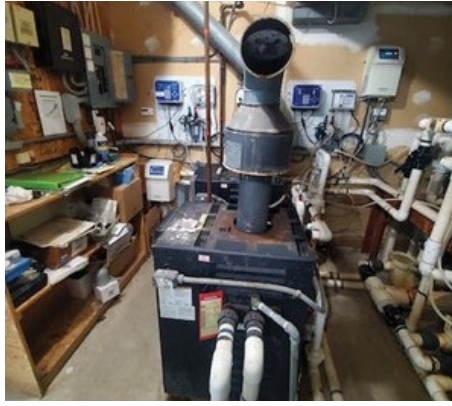
A non-functioning barometric damper, as seen here, is another opportunity for carbon monoxide to escape the flue and enter the occupied space.
