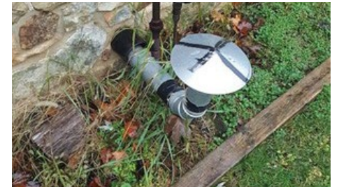
This is a Category 3 appliance that has been vented with incorrect material. Most codes dictate that a vent must terminate at least 18 inches above the proposed snowline. If the vent is blocked by snow, carbon monoxide would back up into the occupied space. Also, the gas regulator, which has a vent, is far too close to the hot surface of the vent termination, which is a potential source for ignition.
