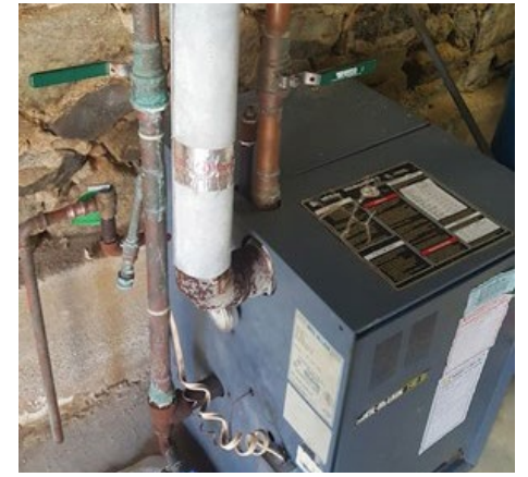
This is a Category 3 appliance that has been vented with incorrect material. Condensate became trapped in the vent elbow and caused deterioration. All photos courtesy Tom Soukup.
